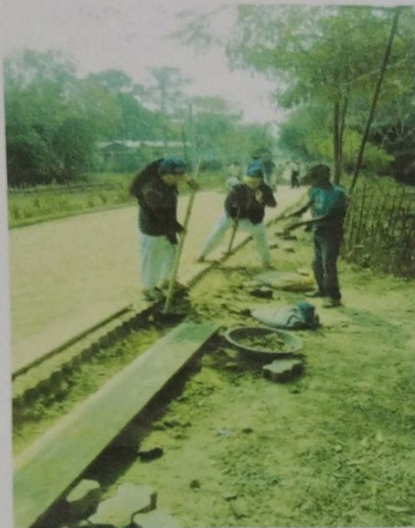
The repairing of a kutchra road due to release of excess water from a residential complex
